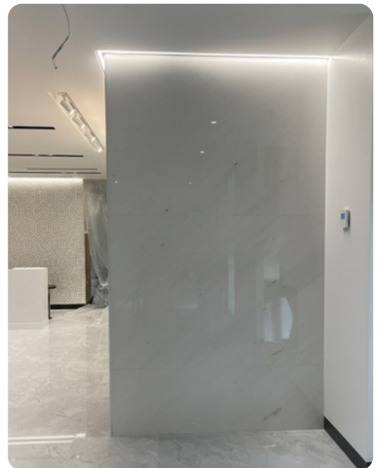
Project : UBS Securities Philippines, Inc. Address : Ayala Triangle Gardens Tower 2, Makati City
